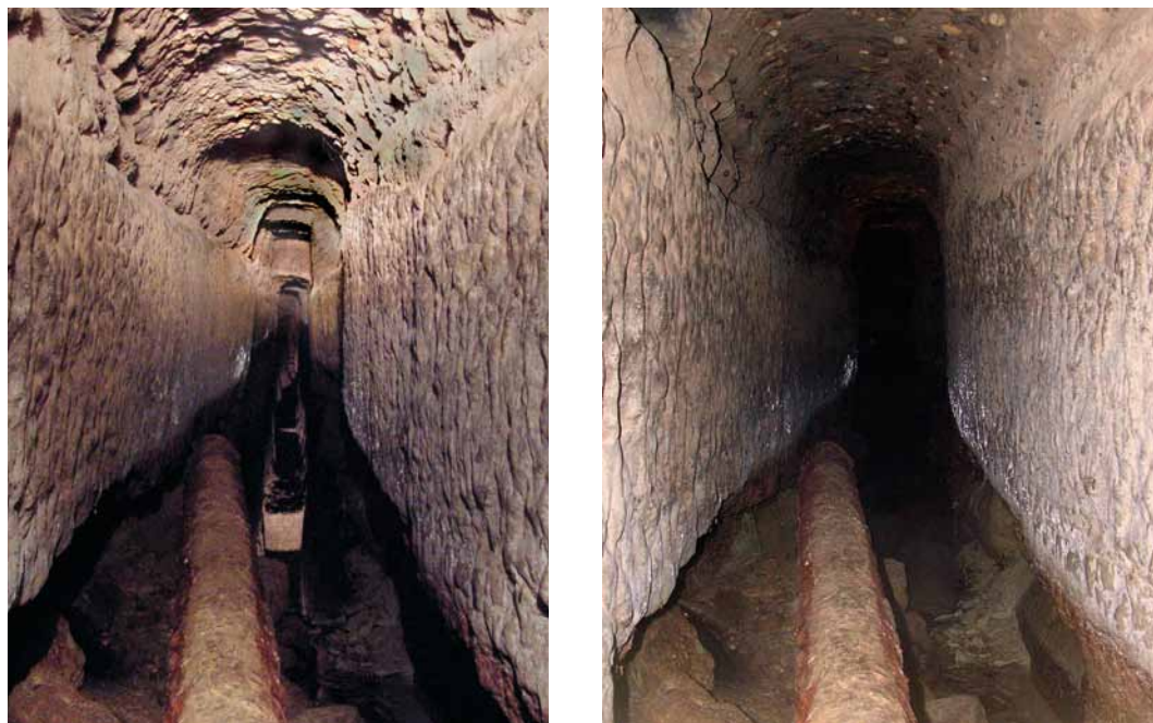
Figure 13. Peirene: East supply tunnel, photographs showing view south from modern dam at Manhole A, with two lighting schemes highlighting conglomerate ceiling, sandstone walls, and change in ceiling height (at back of left image)
